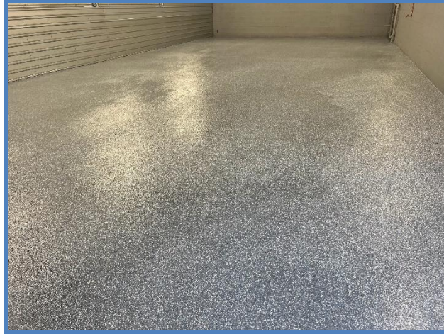
Uneven topcoat on a full chipped floor = Coating Fail!
